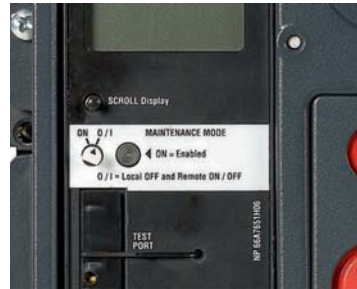
Direct ARMS activation on the circuit-breaker
